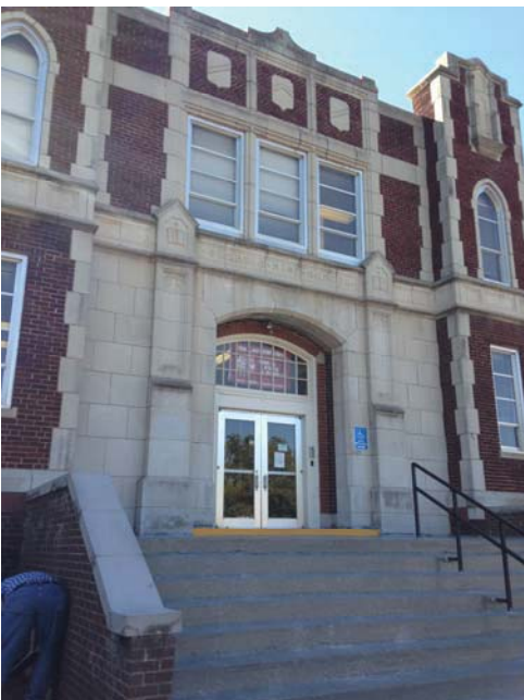
Exterior needs tuckpointing
