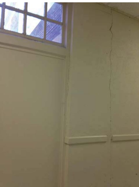
Movement at previous addition line
