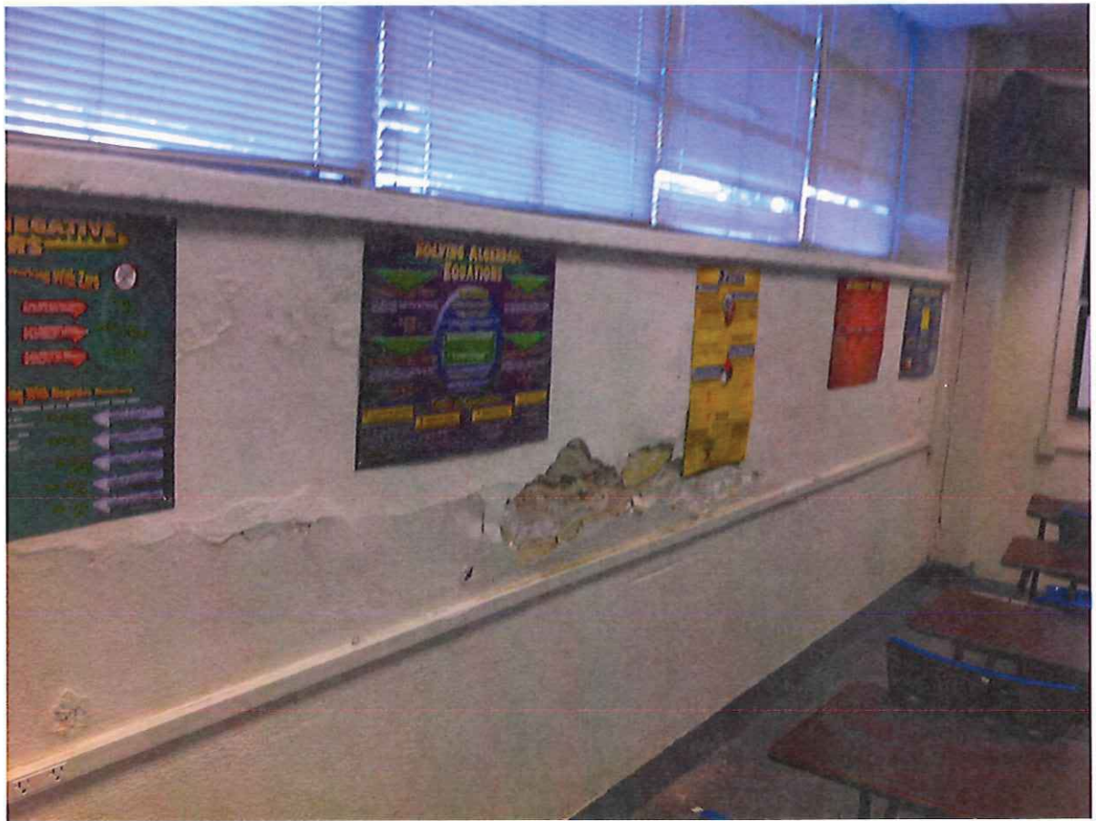
Picture #1 – Water Damage at First Level
