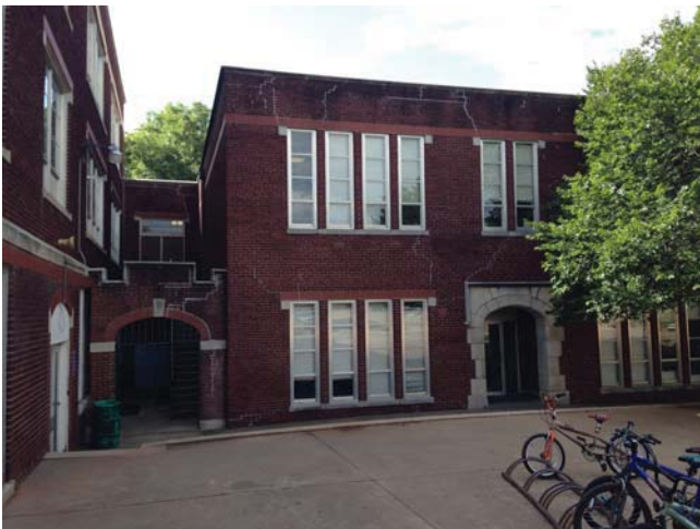
Brick needs tuckpointing
