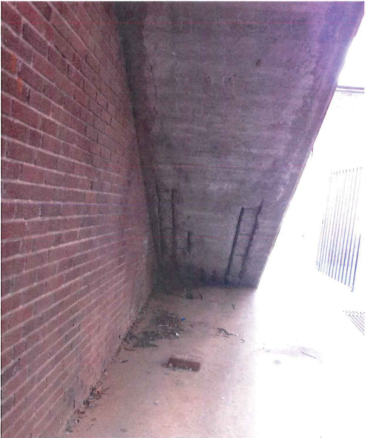
Picture #12 – Exposed Reinforcing on Bottom Surface of Exterior Stair
