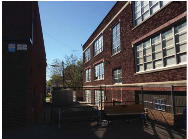
All windows should be replaced
