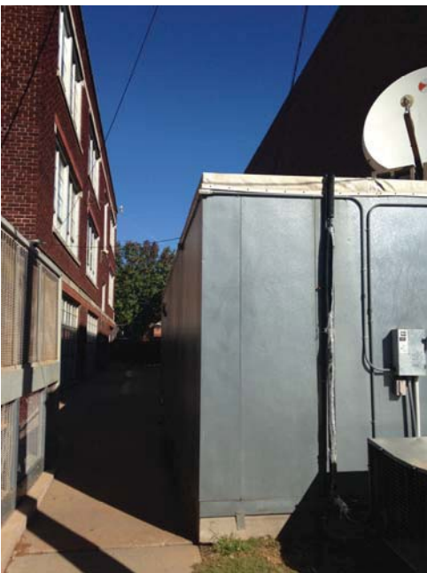
Cooler/ freezer located outside
