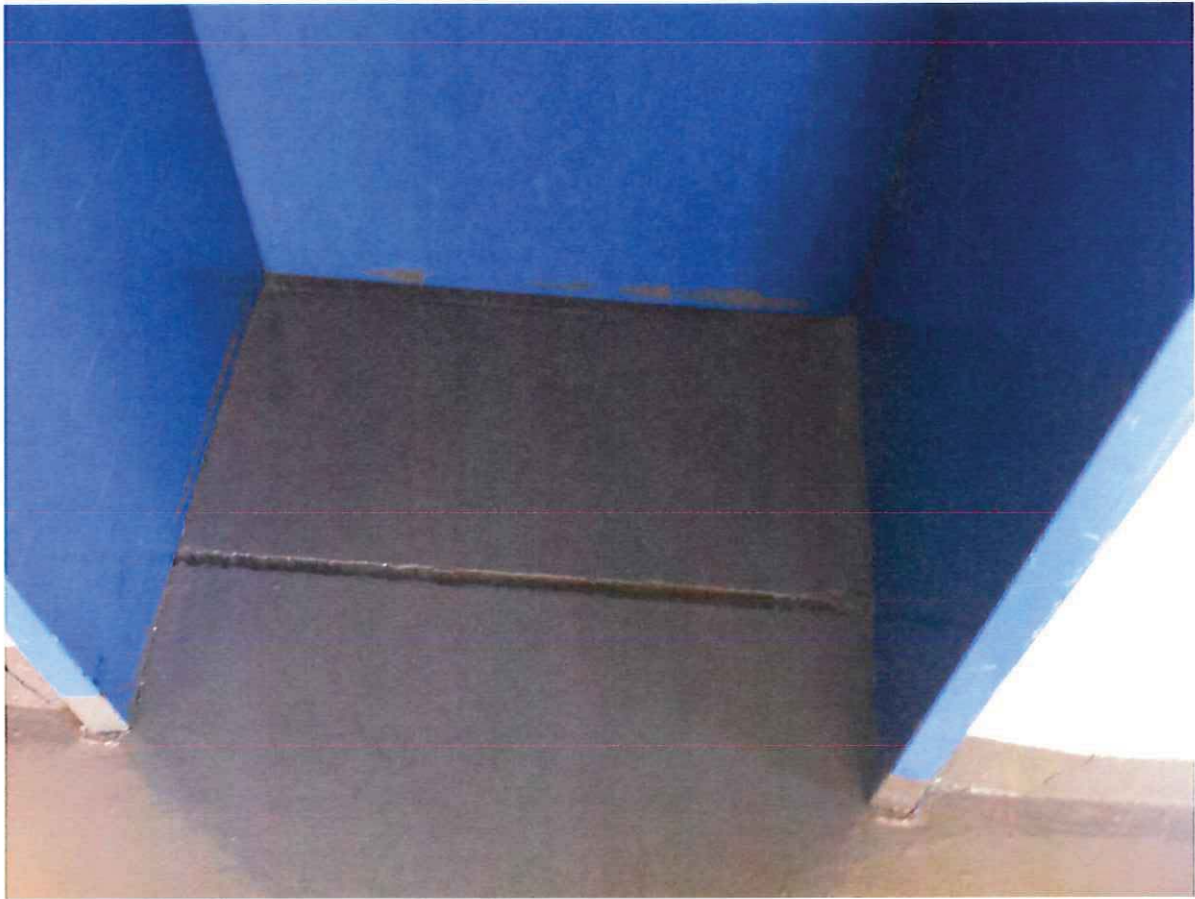
Picture #7 – Separation at Threshold of Elevator at Third Level
