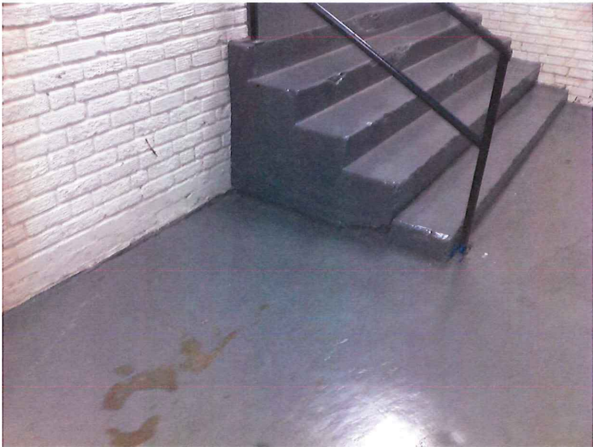
Picture #5 – Settlement at Base of Stairs to Shop Classroom
