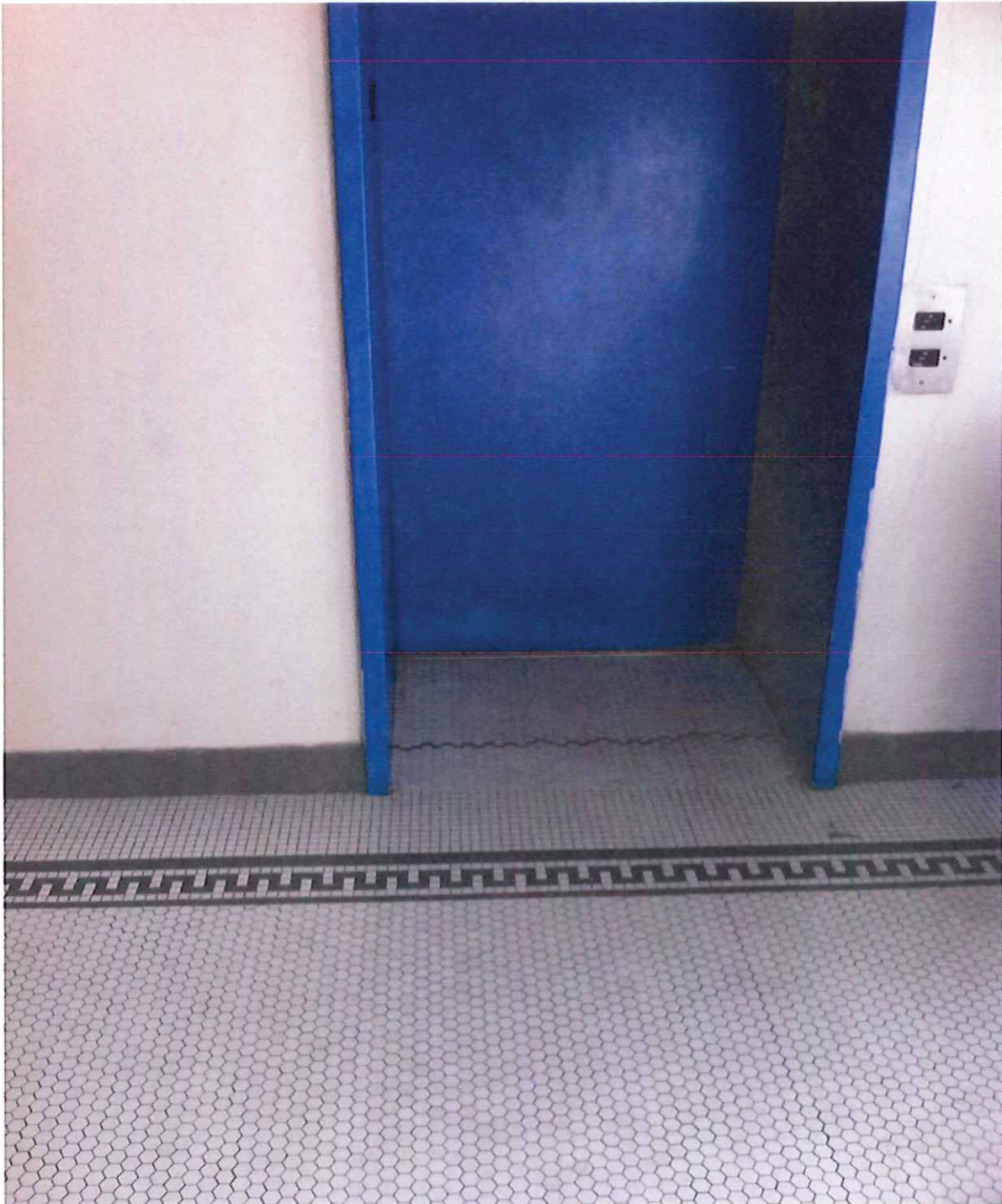
Picture #6 – Separation at Threshold of Elevator at Second Level
