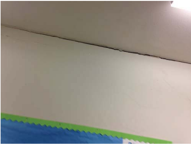
Some settling observed—easily corrected
