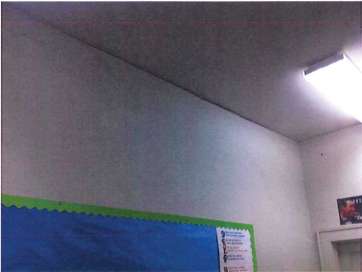
Picture #4 – Settlement Crack Between Wall and Ceiling in Storage Room
