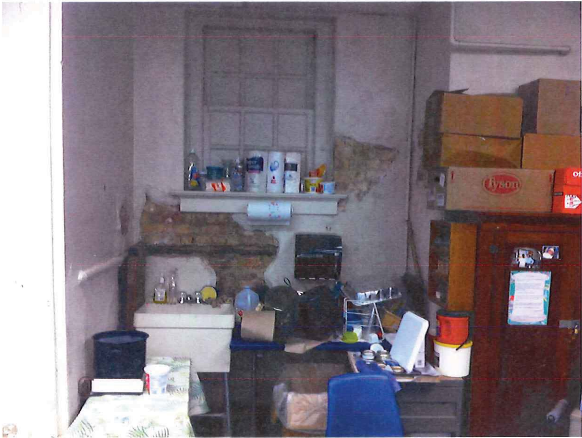
Picture #3 – Water Damage at First Level
